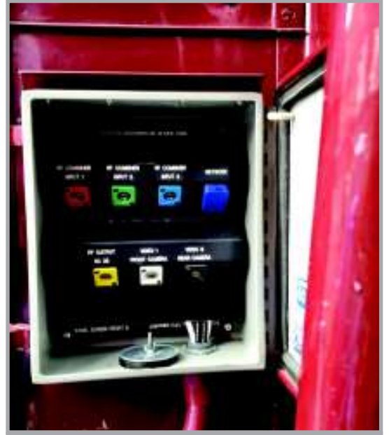
This typical junction box, located on each of the four outside corners of the cars, provides interconnection for audio, video, RF distribution and network.
